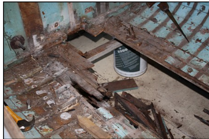
The extent of deterioration is obvious here . . .
